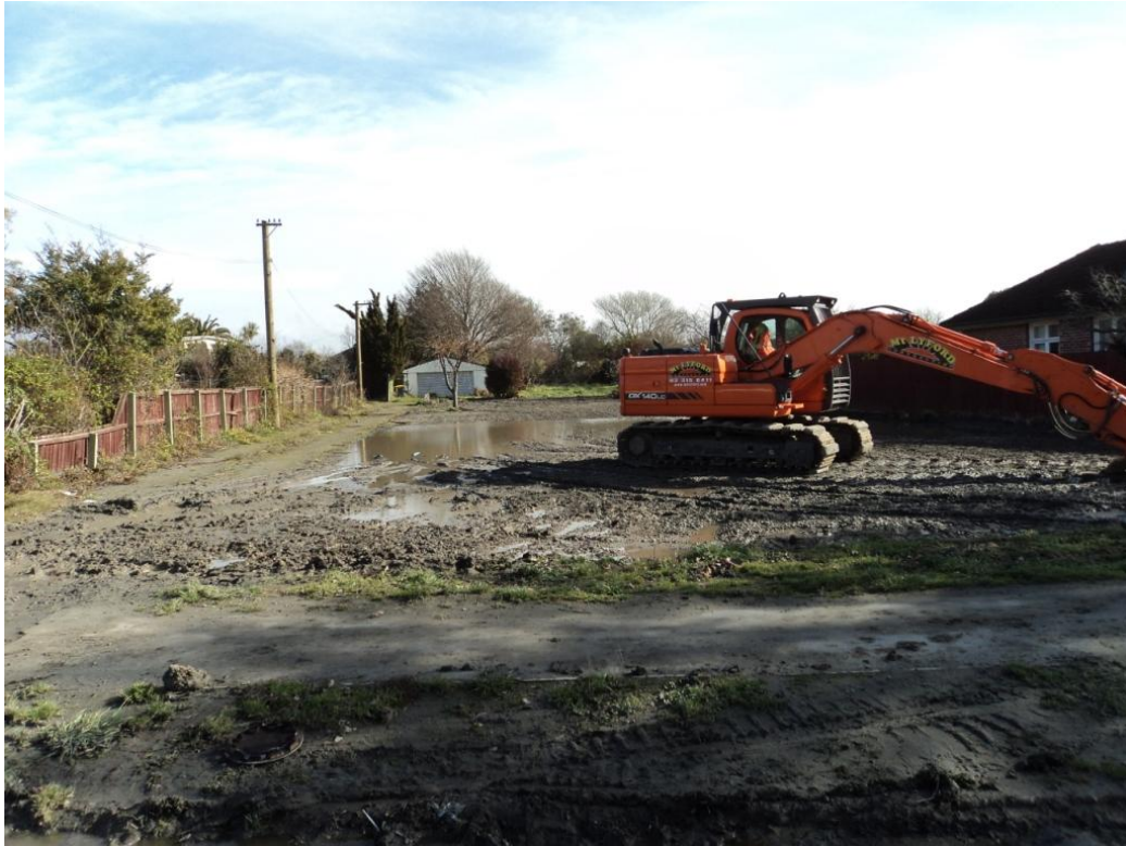
Figure 2: Surface flooding extending across property boundaries – 189 New Brighton Road, Burwood, 3 August 2012
